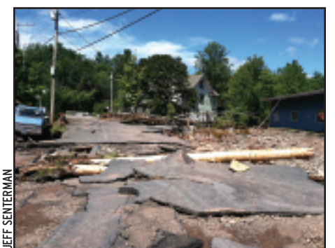
Washed out roads and bridges, such as this road in Tannersville, NY, are the biggest obstacles to full trail access in some areas.
