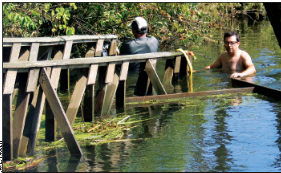
Frank Dogil, Bob Haas and Steve Klauck (not shown) reset the Swamp River AT bridge in Pawling, NY.
