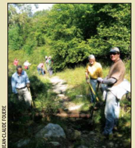
Volunteers turned out for a work trip to repair storm damage at Minnewaska State Park Preserve.
